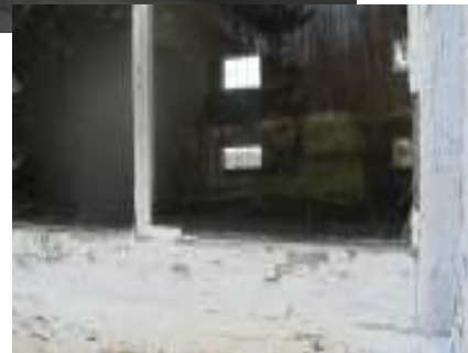
Rotting window frames with missing putty
