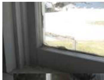
Broken window with glass patch taped on
