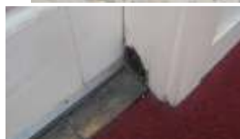
Rotting door frame and sill, plus ill fitting non-weather-tight blue entry door
