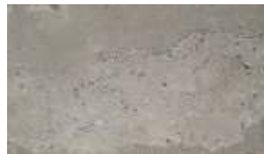
Spauling concrete walkway
